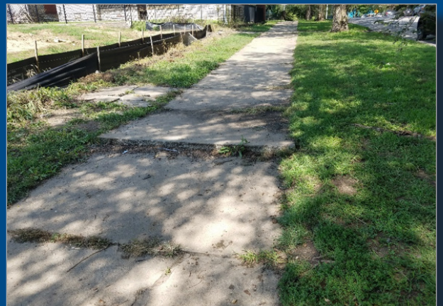
Figure 40: Cleveland Ave, at 9th Street (eastside) Looking North - No ADA Ramps
