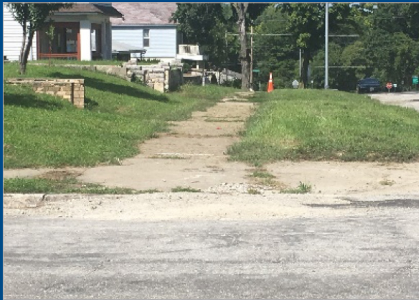
Figure 39: Prospect, westside Looking North from Garfield Elementary School - No curb or ADA accommodations
